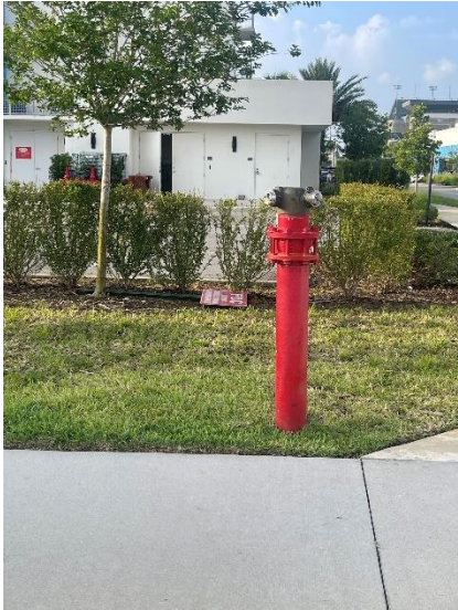
For informational purposes Maintenance (Replace FDC Sign) Location: Corner of Legends Lane & drive between parking garage and Icon Apartments
