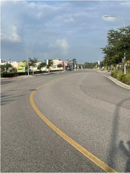
Faded Striping Location: Legends Lane
